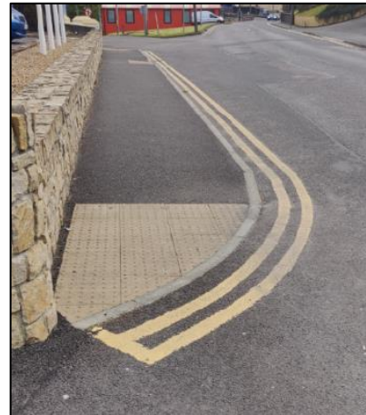
Figure 2-6: Existing tactile paving not reinstated
