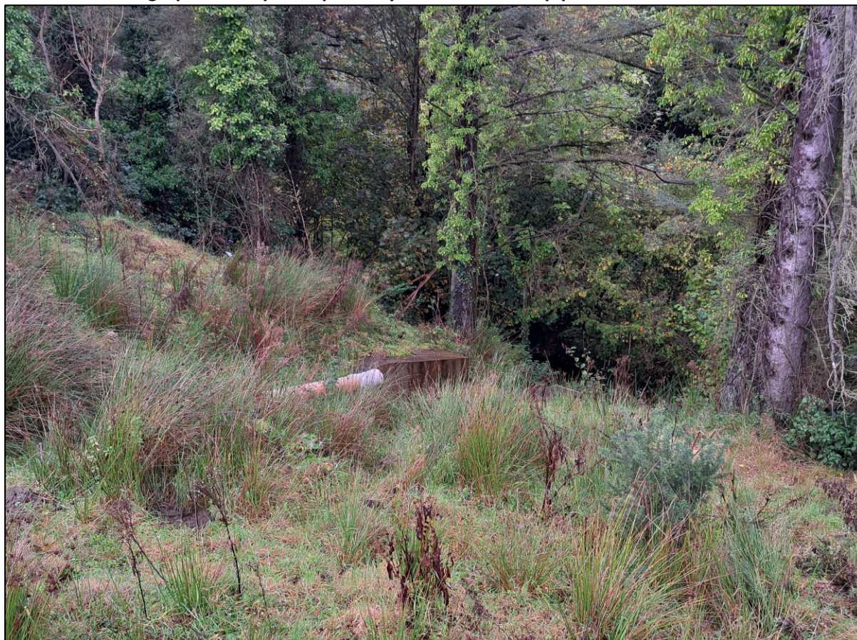
Photograph 4.3: Impeded pathway from the outfall pipe to the Malin Stream.
