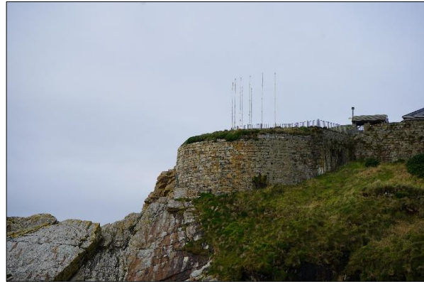
Plate 3.6: Lower Fort – Lough Swilly Walkway to be constructed on the seaward side of the fort [January 2023]
