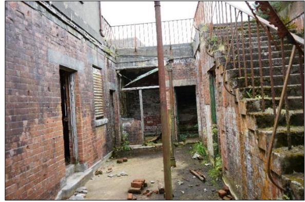
Plate 2.43: PRA – the brick structures at the high fort were assessed as being of low suitability for roosting [August 2023]
