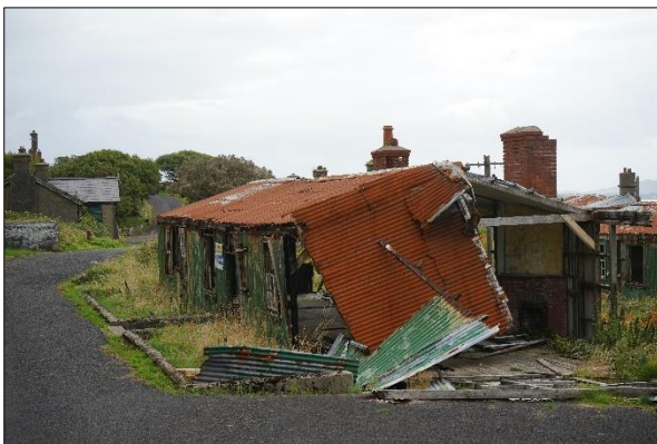
Plate 2.36: PRA – the cluster of derelict barracks/billets buildings; all assessed as being of negligible suitability for roosting [August 2023]
