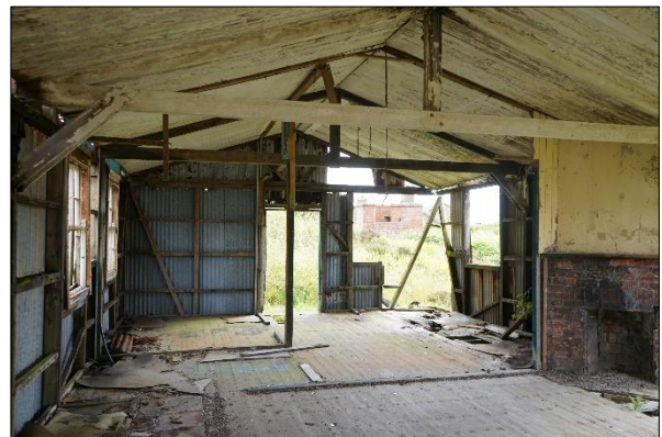
Plate 2.37: PRA – view of the interior of one of the more intact timber and metal sheeting barracks/billets buildings [July 2022]
