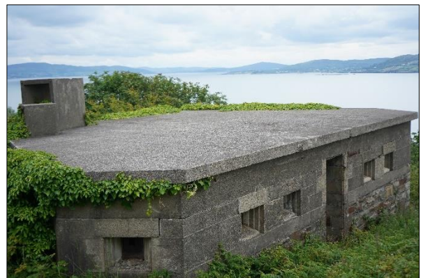
Plate 2.38: PRA – typically small and low solid concrete structure; all assessed as being of negligible suitability for roosting [June 2022]
