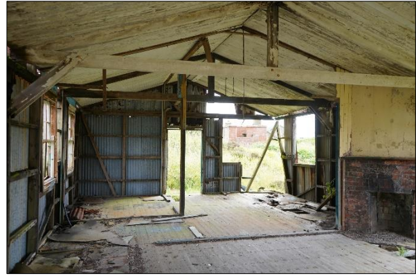
Plate 3.16: Billet Buildings – typical view of the interior or the derelict billet buildings [July 2022]
