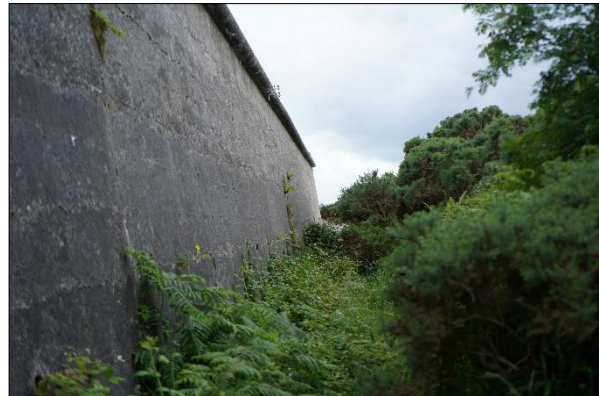
Plate 3.3: High Fort / Redoubt – gorse-dominated scrub and dense bracken will be lost from around the exterior [June 2022]
