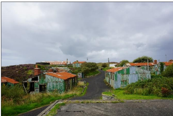
Plate 2.35: PRA – the cluster of derelict barracks/billets buildings; all assessed as being of negligible suitability for roosting [August 2023]
