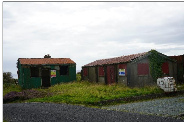
Plate 3.14: Billet Buildings – typical view of the derelict billet buildings and surrounding vegetation & hard-standing [August 2023]
