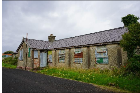
Plate 3.18: Brick Buildings – 1 of 2 adjacent buildings to be restored and repurposed as Welcome Buildings [August 2023]
