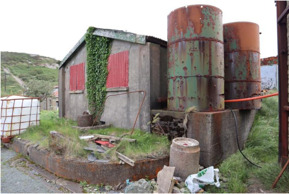
Figure 105 – 18.02 Fuel & Cooling Tanks
