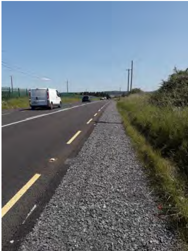
Plate 15. Looking east on approach to Ballyshannon, grassy verge, hedgerow and surface water drainage percolating to ground.
